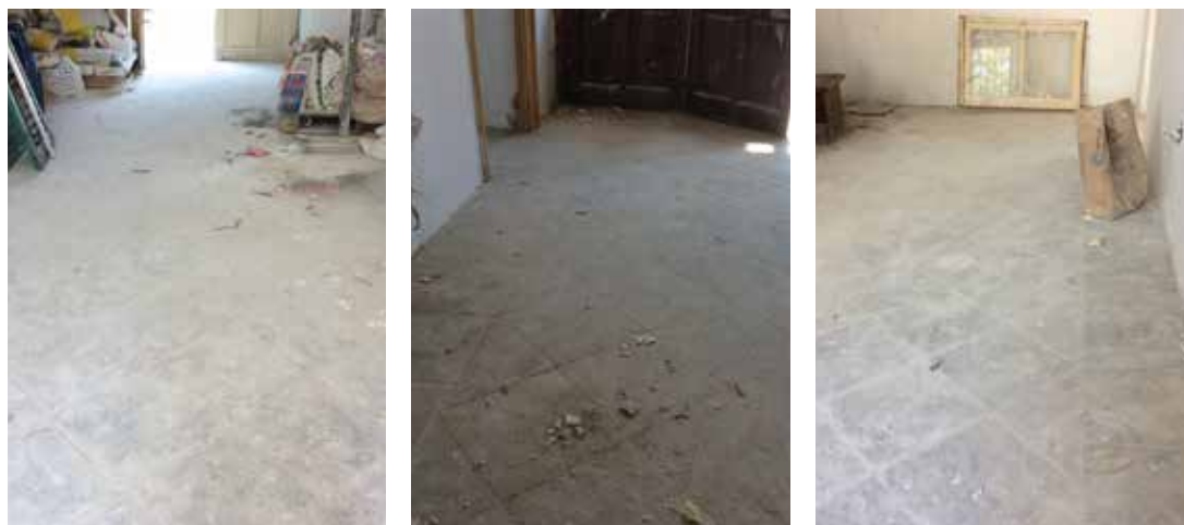
Figure 15a/b/c: Condition of Cyprus marble floors on the ground floor and preparatory works before restoration: Entrance hall (Menteş, 2016)
